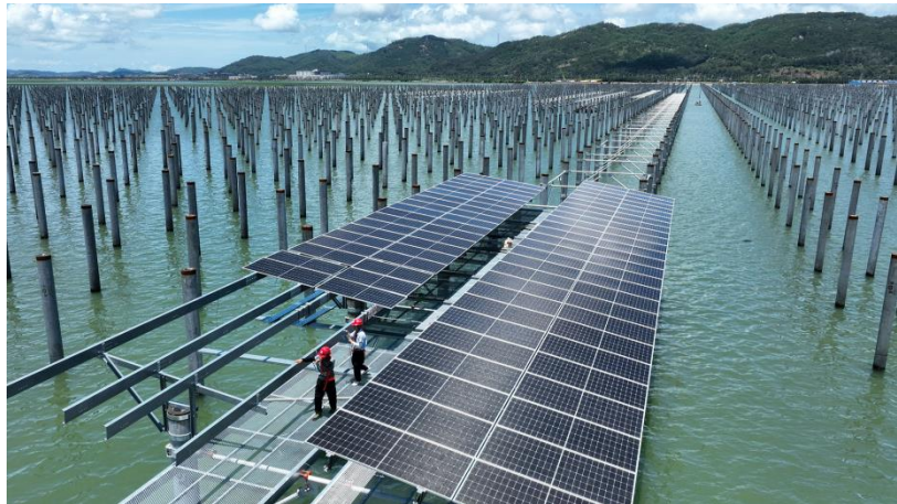
14 In this undated file photo, technicians install photovoltaic panels at a solar power farm in Dongshan county, Fujian province. (PHOTO / XINHUA)
